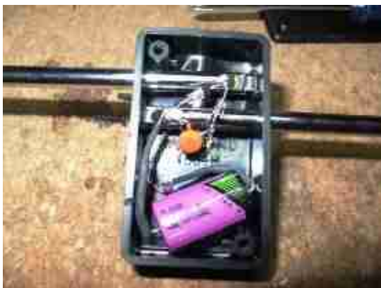
Inside Wiring View
